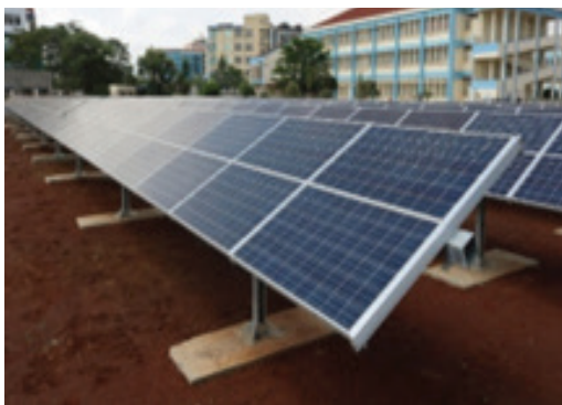
Figure 38: A photo of Kenyatta University Solar Power Plant
